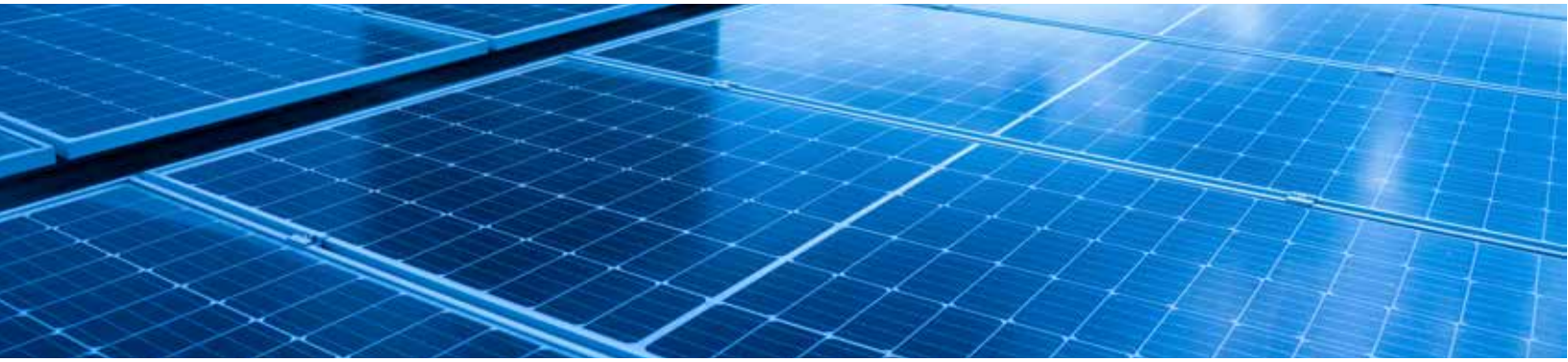
Photovoltaic modules in solar panels
